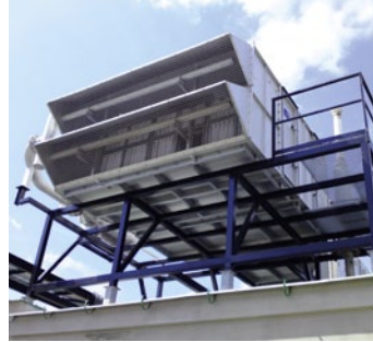
Filter suction system
