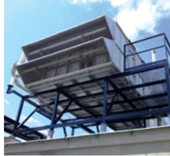
Filter suction system
